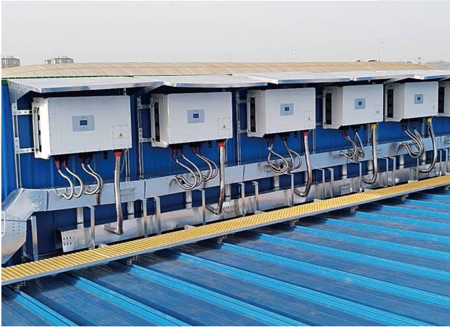
China ▶ Inverter: SUN-110K-G Capacity: 660kW
