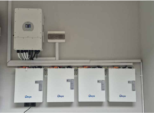
Indonesia ▶ Inverter: SUN-12K-SG Capacity: 12kW/20kWh
